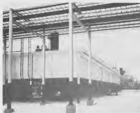
VIEWED FROM the road, one of the most striking pieces of construction huge bank of air fin coolers, above. Antilles will make use of salt water also in controlling process streams. Gas purification vessels, right, front a section of the ammonia plant. This series of vessels achieves the removal of bon monoxide and carbon dioxide. These carbon toms must be removed to the isolation of hydrogen and nitrogen necessary for eventual ammonia synth. The carbon removal stage is after hydrogen generation and before compr
